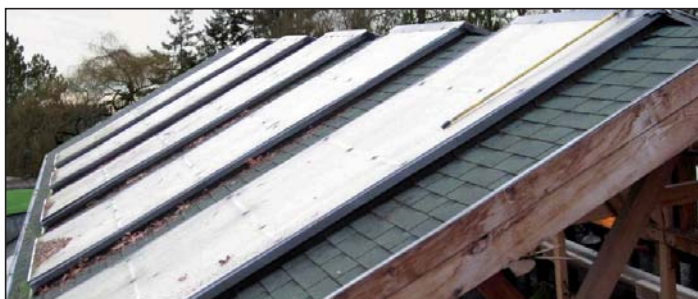
Before: Deteriorated leaking skylights caused extreme glare and heat build-up.
